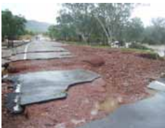
Roads were ripped apart
