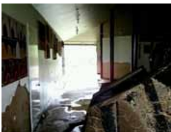
Damaged Warmun Arts Centre
