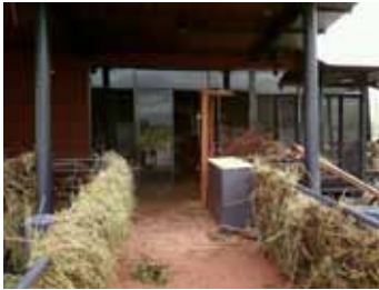
Damaged Warmun Arts Centre
