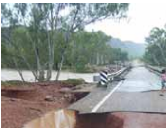
Roads were ripped apart
