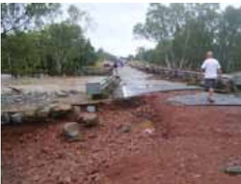
Roads were ripped apart
